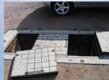
(Grease Arrestor Pits)
